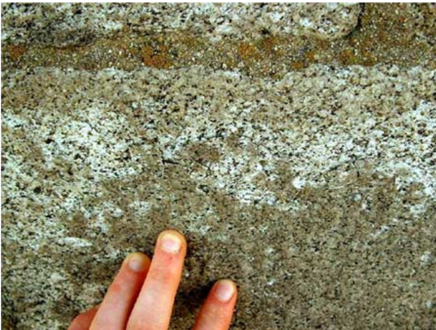
Fig. 12: efflorescence and sugaring on a granite ashlar wall block, Aberden (Great Britain).
