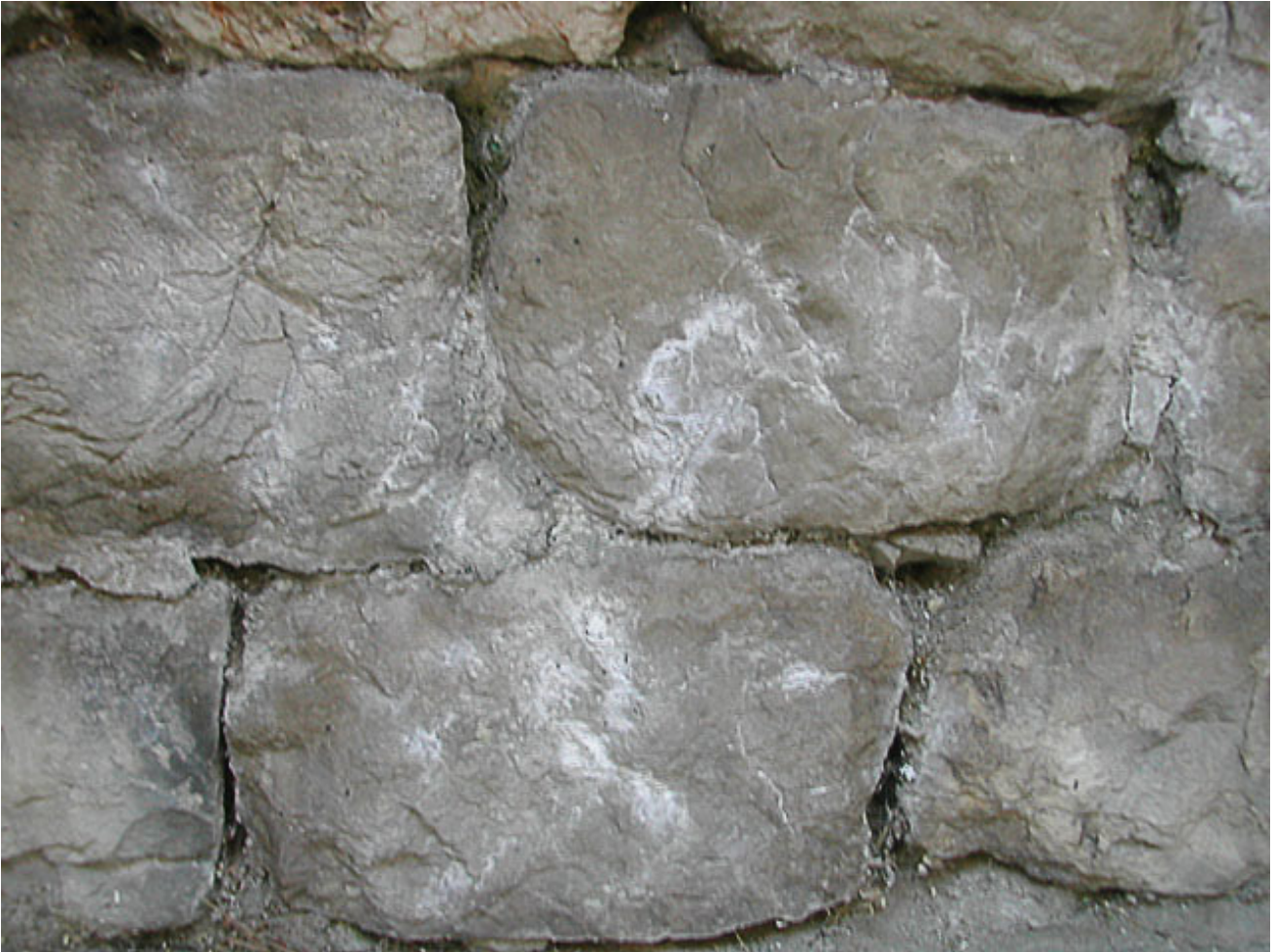
Fig. 2: limestone blocks' surfaces deteriorated by salt crystallization cycles, Dubrovnik (Croatia).
