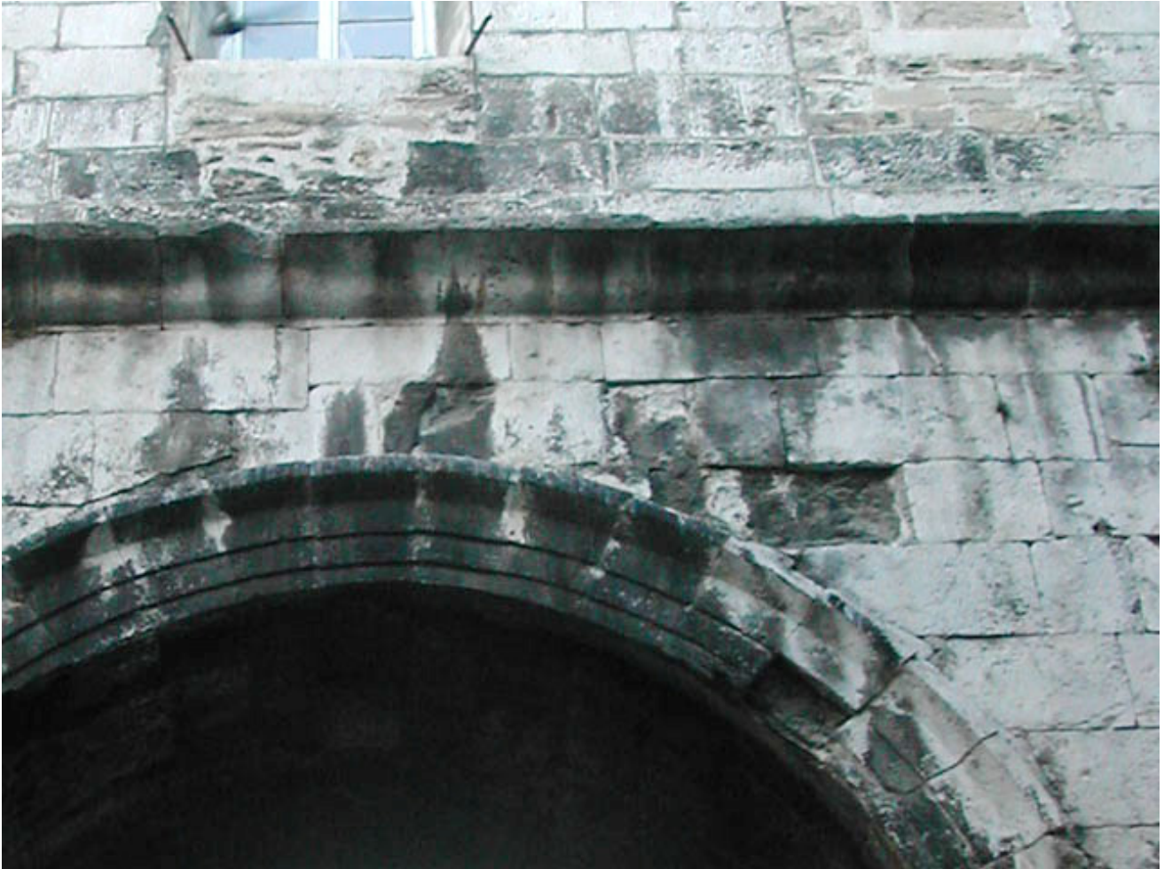
Fig. 3: signs of intense sulphatation outcomes on white limestone architectural details, Diocletian Palace, Split (Croatia).
