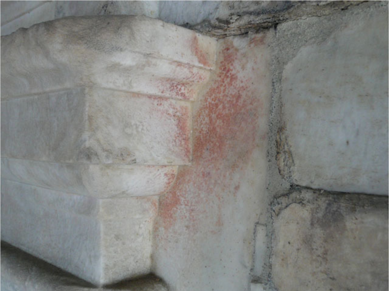
Fig. 11: red stains produced by lead resistant bacteria growing on marble's architectural detail surface, Florence Cathedral dome (Italy).
