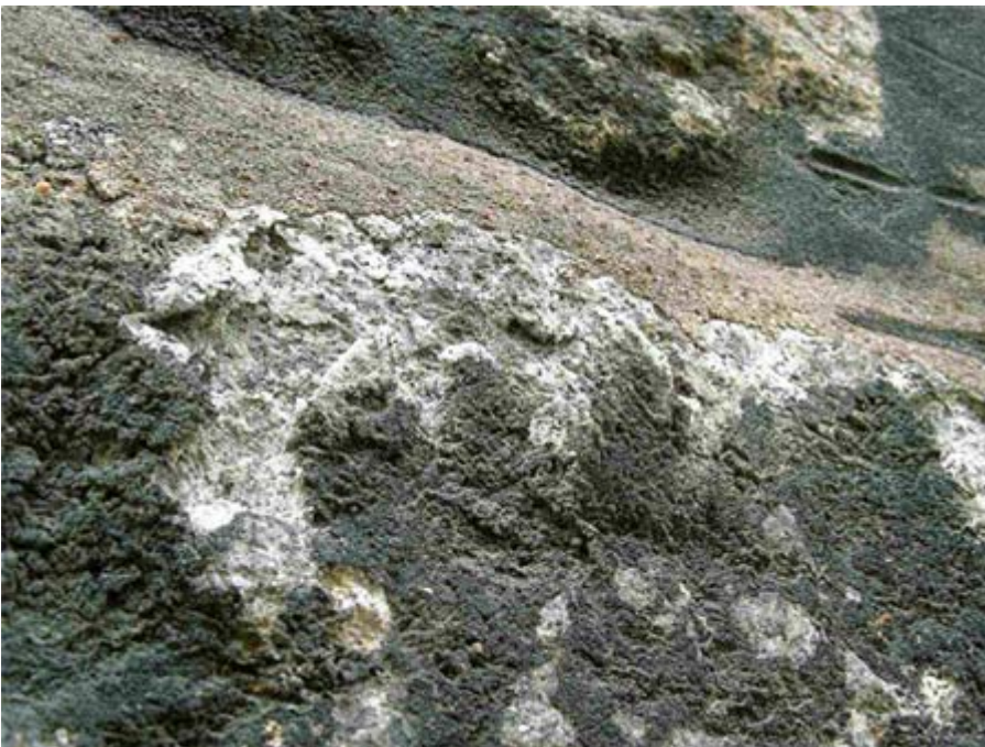
Fig. 14: sulphatation and black crusts on a granite ashlar wall block, Aberdeen (Great Britain).
