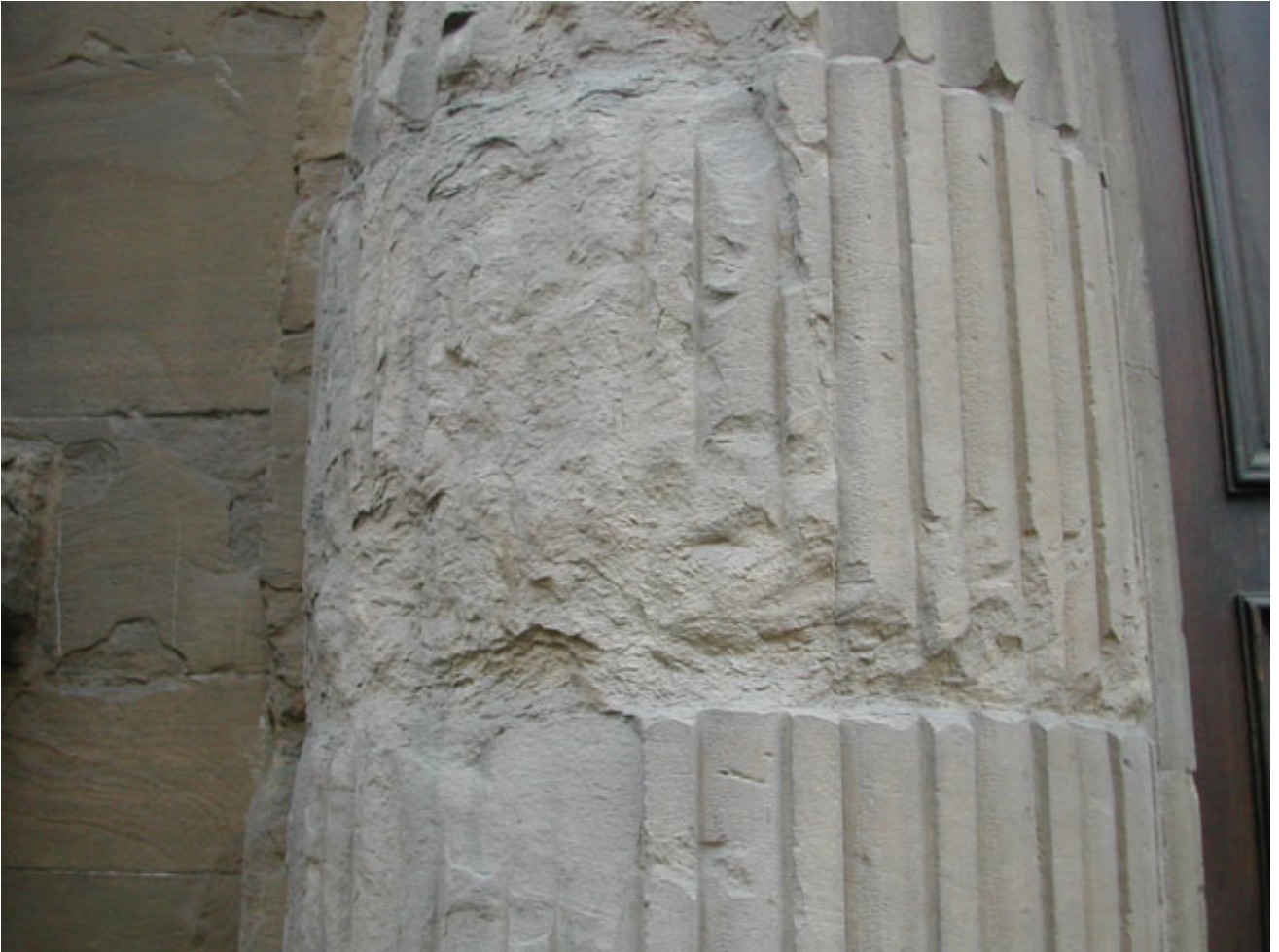
Fig. 1: clear signs of water crystallization effects on northern face of a sandstone column section, Florence (Italy).
