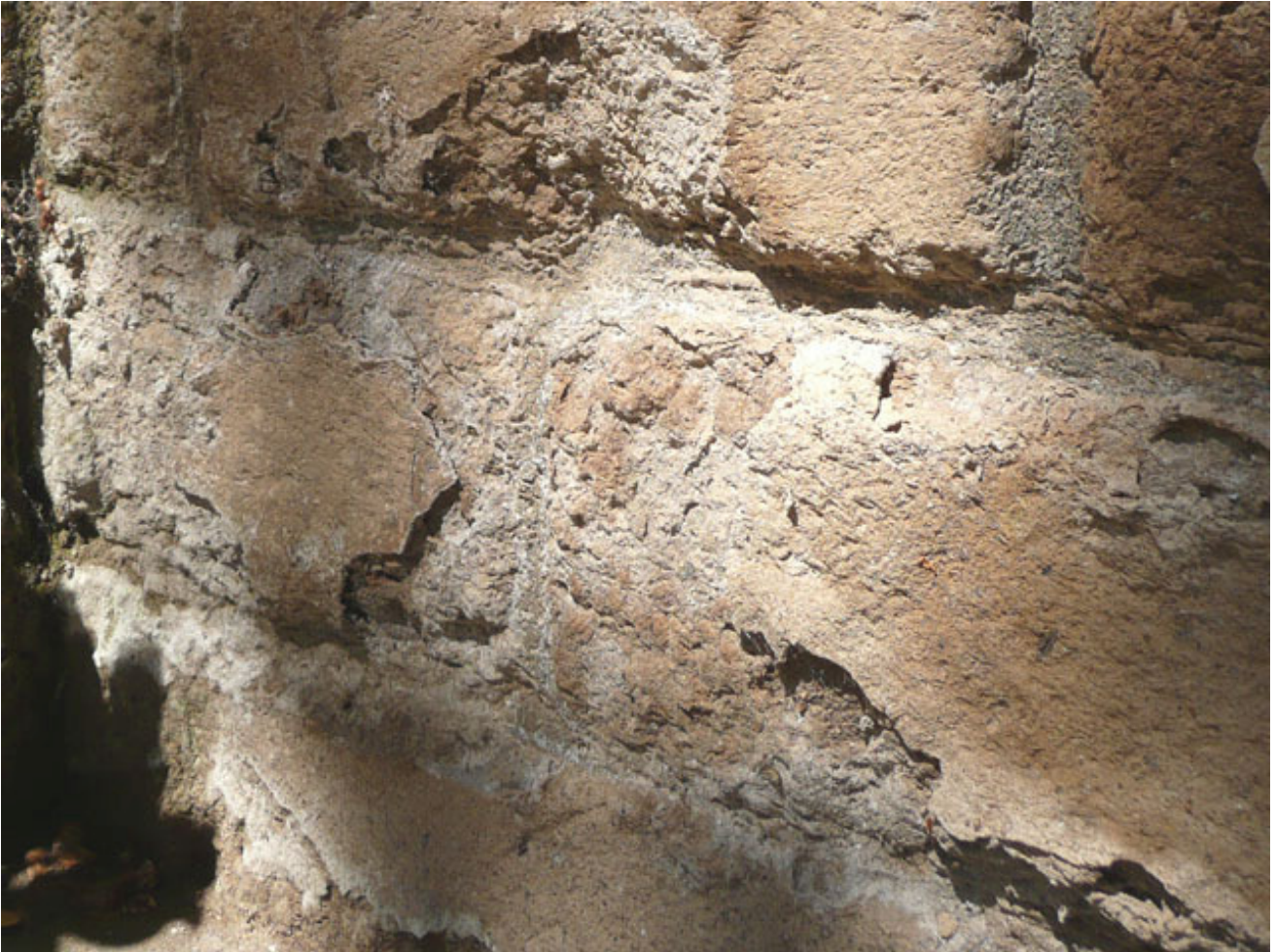
Fig. 13: sub-efflorescence leading to extreme bulging and spalling of tuff ashlar wall blocks, southern Tuscany (Italy).
